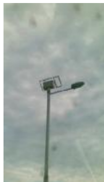
Figure 1: Fixed Solar Panels for Lighting Gaza Valley way
