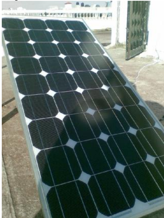
Figure 7: Solar Module mounted on Home Roof
