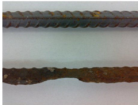
Figure (7): Corroded and Non-corroded steel reinforcement bars
