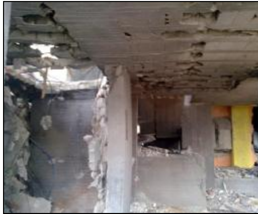
Figure (5): Buckled ground floor column
