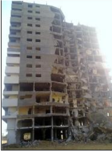
Figure (3-a): Damages in the western side
