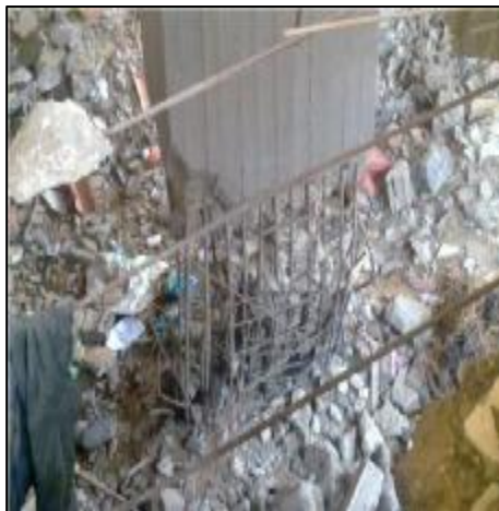
Figure (4): Column showing severe damage
