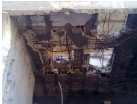
Figure (7): Limited damages in ground floor slab
