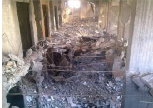
Figure (6): Part of the destroyed basement slab
