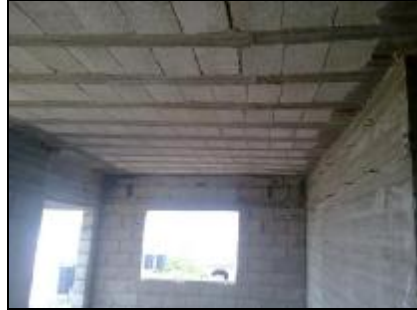
Figure (8): Excessive deflection of a panel in second floor slab around column C11
